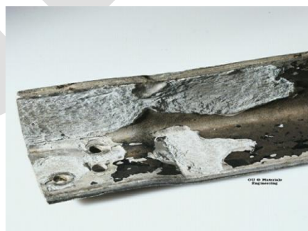
Figure 1.2 Effects of salt corrosion problems
