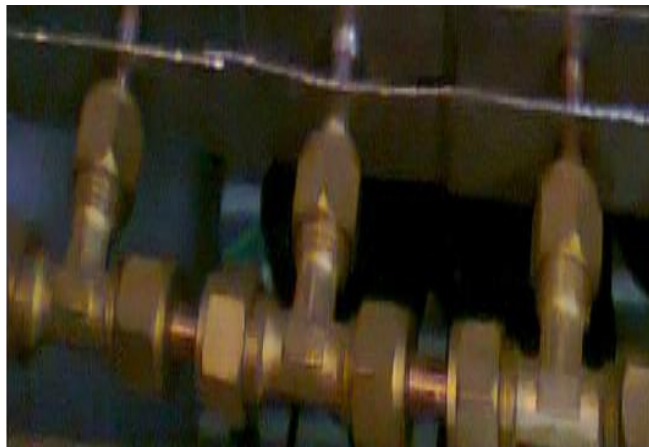
Fig. 1 Main steam pipe
